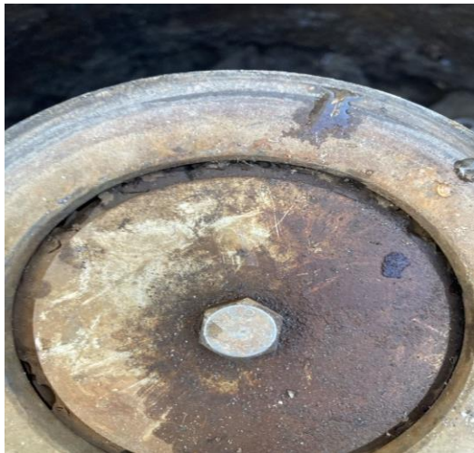
VAPOR RECOVER ADAPTER NEEDS REPLACED ON PUL TANK - DAMAGED
