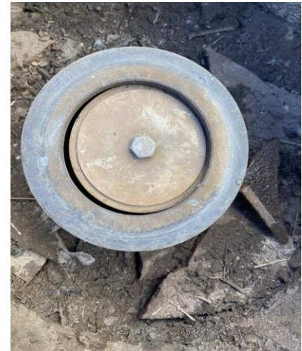
VAPOR RECOVER ADAPTER NEEDS REPLACED ON RUL SLAVE TANK
