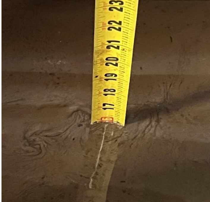
DISP 1/2 SUMP TEST END 16"
