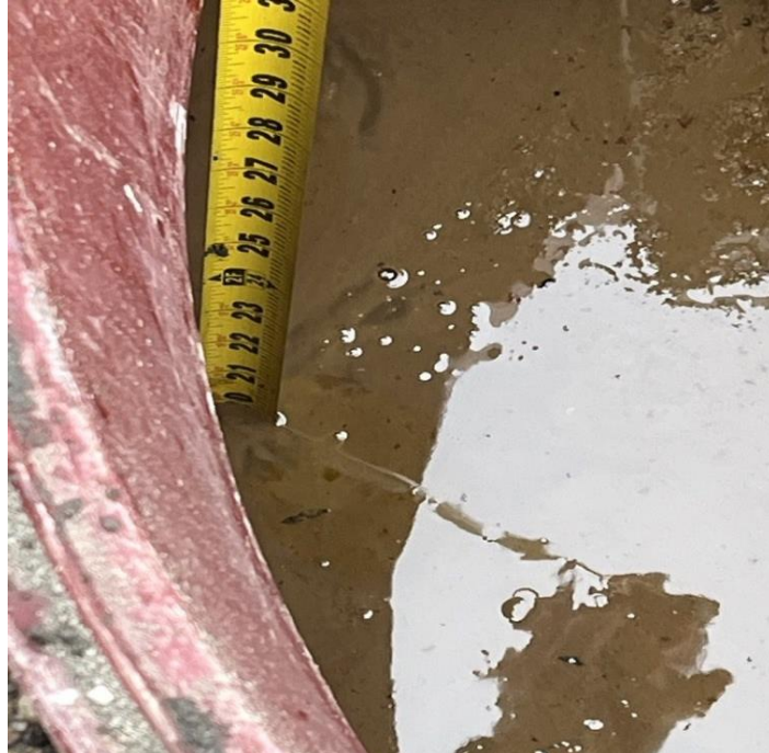
KER STP SUMP TEST END 20"
