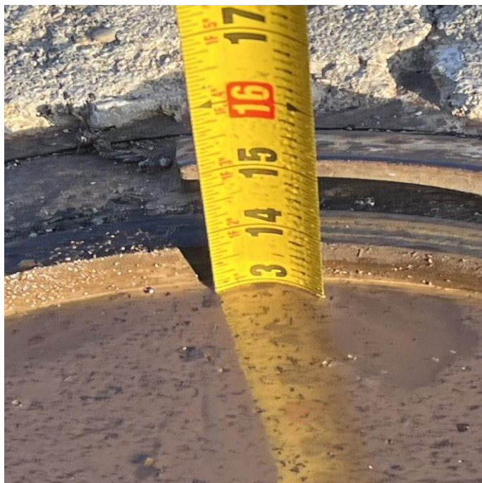
RUL SPILL BUCKET TEST START 13"
