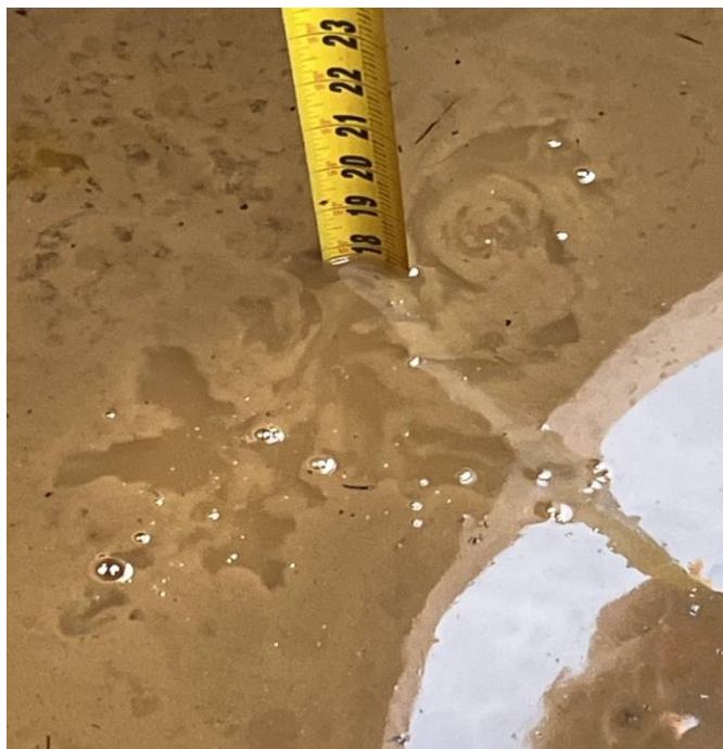
DSL STP SUMP TEST START 17.75"
