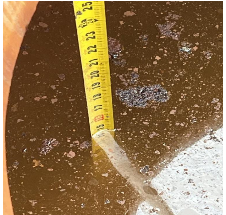
RUL STP SUMP TEST END 15"
