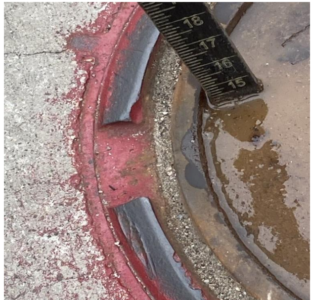
PUL SPILL BUCKET TEST START 14.5"
