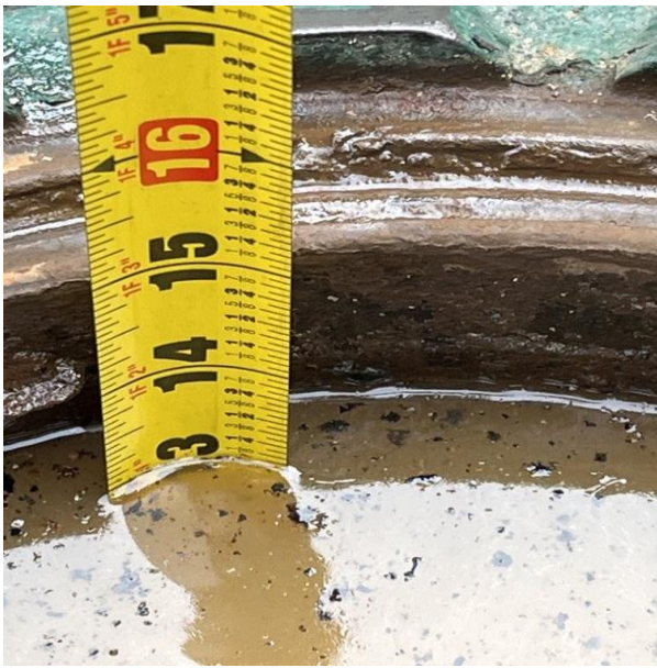
DSL SPILL BUCKET TEST START 13"
