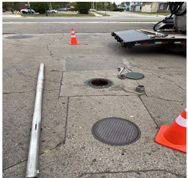
NO DSL OVERFILL POSSIBLE BALL VALVE BUT NOT ACCESSIBLE TO VERIFY
