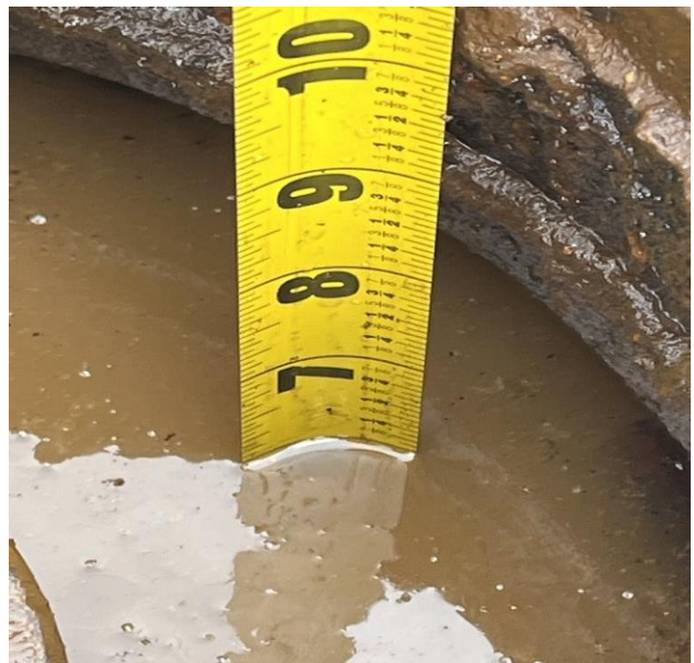
RUL1 SPILL BUCKET IMMEDIATE FAIL - FROM 10.5" TO 6" WITHIN 30 SECONDS
