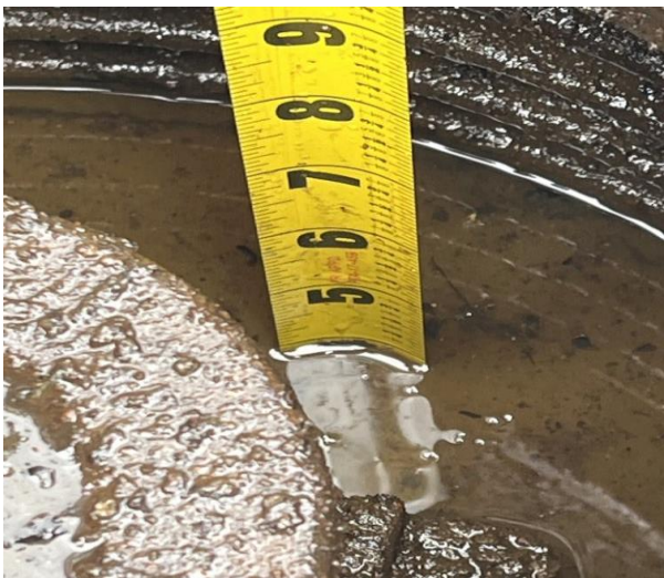
RUL2 SPILL BUCKET IMMEDIATE FAIL - FROM 12" TO 4" WITHIN 30 SECONDS
